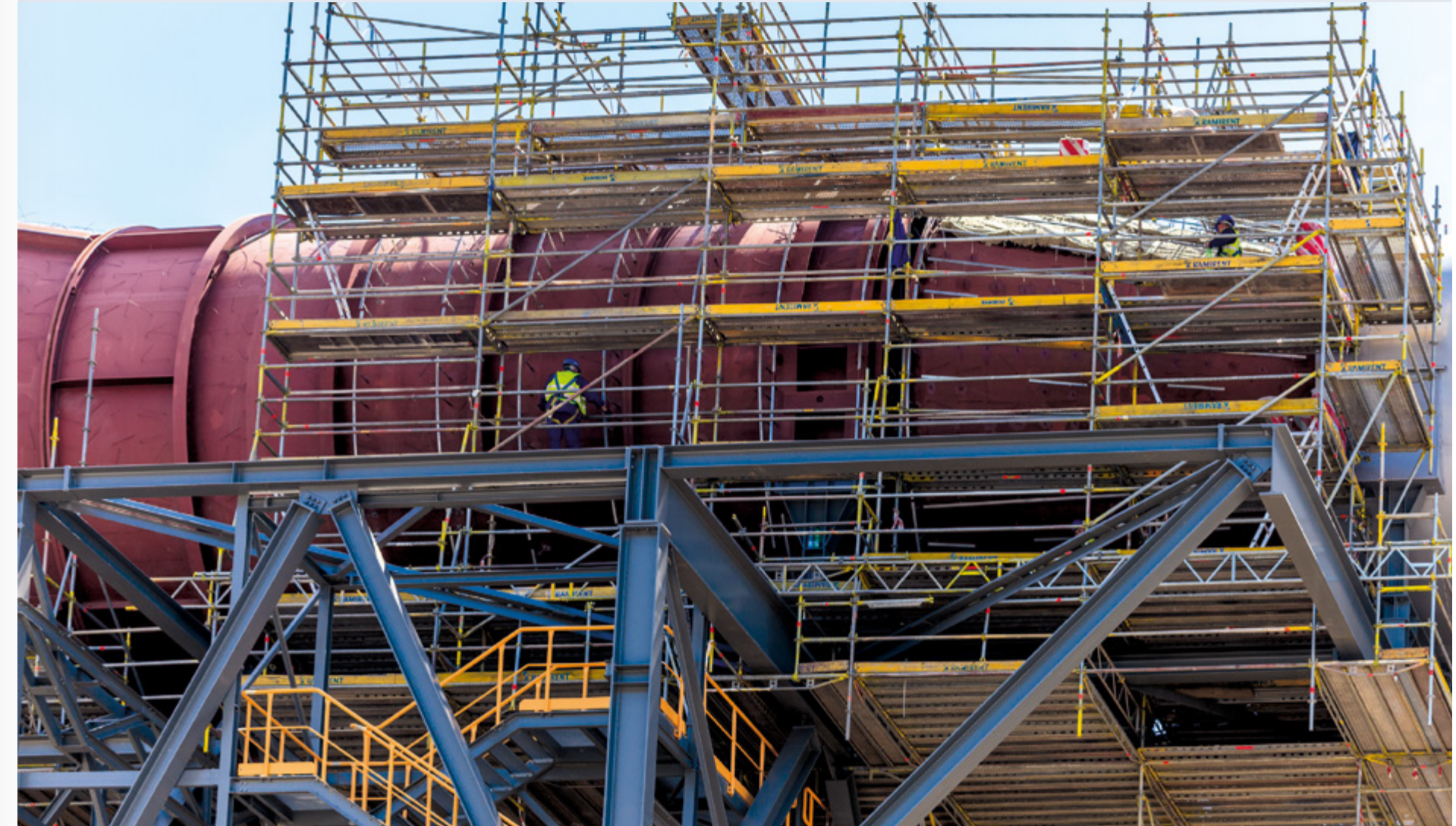
PERFORMANCE OF COMPLEX CIVIL WORKS FOR WET-FLUE GAS DESULPHURISATION PLANT AT RYBNIK POWER PLANT
