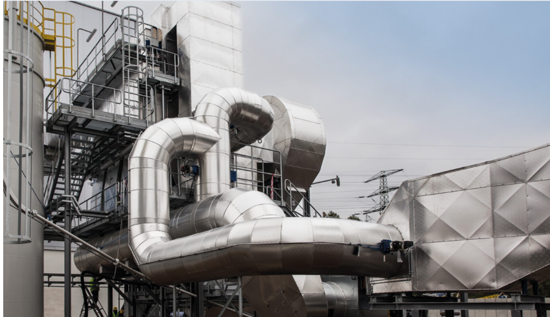
CONSTRUCTION OF A BOILER HOUSE WITH WR-25 BOILER AT MIECHOWICE CHP PLANT
